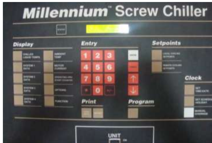
Figura 45. Tablero de control Chiller C.H.
