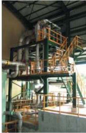
Gas removal system
