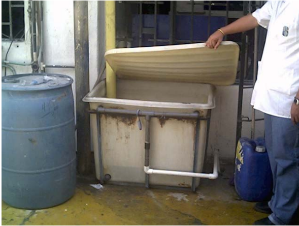
Tanque Recolector M0. (Primer piso)
