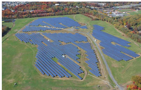
Figura 13. Sistema de paneles solares fotovoltaicos sobre el relleno sanitario de Cuyahoga County, Estados Unidos. Tomado de Solar builder mag Recuperado de https://solarbuildermag.com/news/details-on-the-largest-landfill-solar-project-in-ohio-now-being-constructed/
