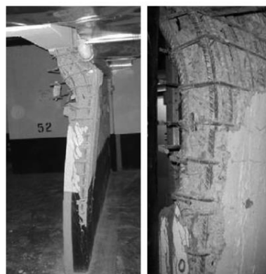
Wall lateral instability.
