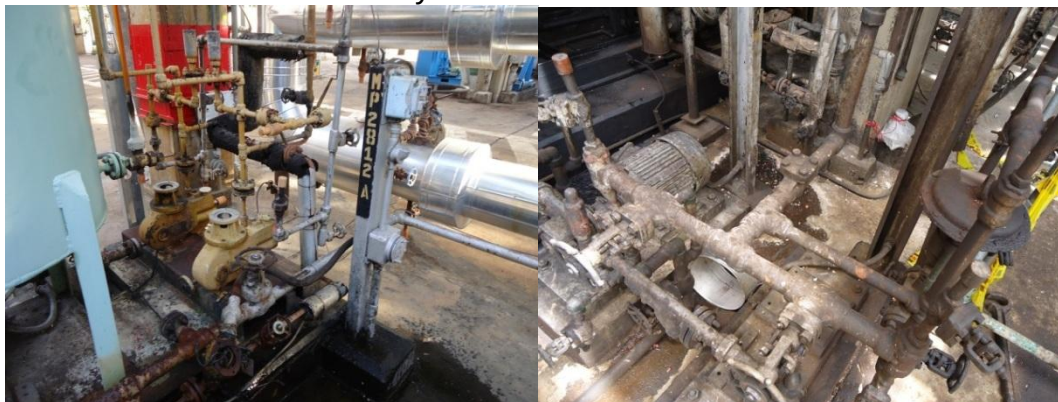
Figura 76. Bombas MP2812A/B y MP2513A/B
