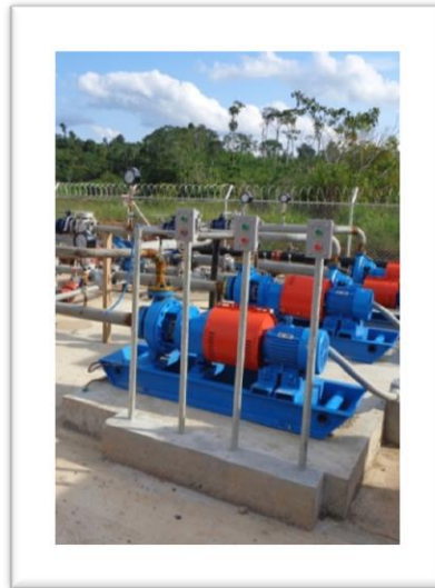
Figura 8. Bombas booster PIA Cohembí 6.
