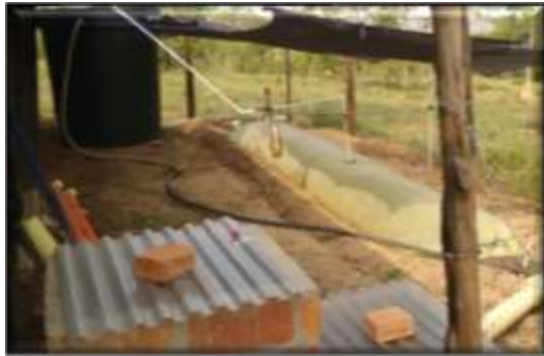
Biodigestor finca Marcella
