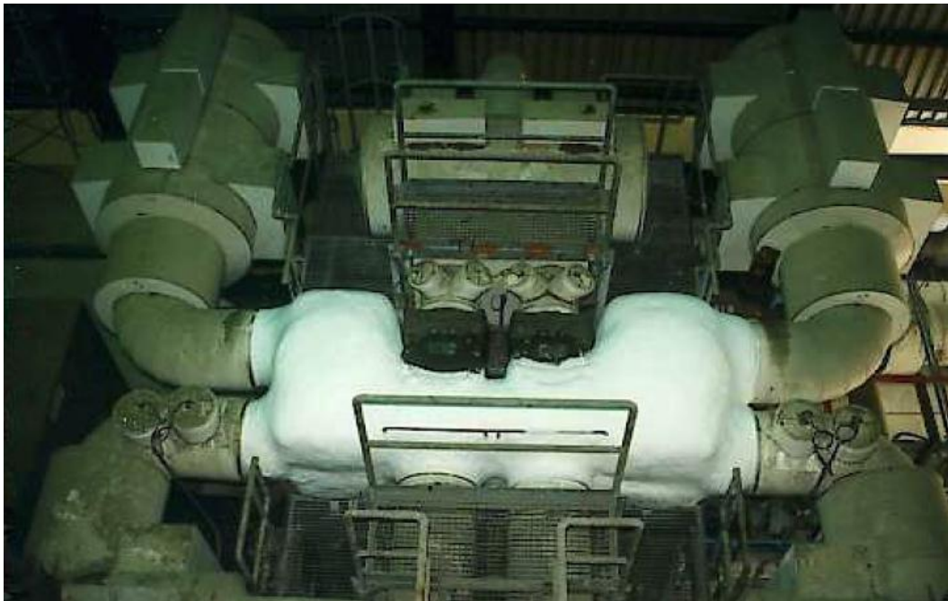
Figura 6. Compresor de boil off gas (BOG)
