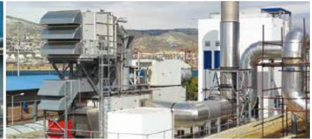
Sewage-sludge drying plant for the City of Athens, on Psytalia island.
