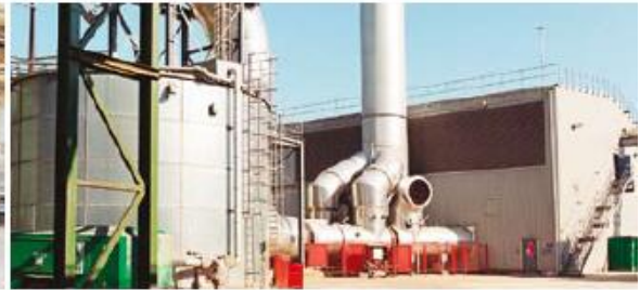
Two SGT-300 gas turbines provide Norbord with electricity and heat at their board manufacturing plant in Scotland, UK.
