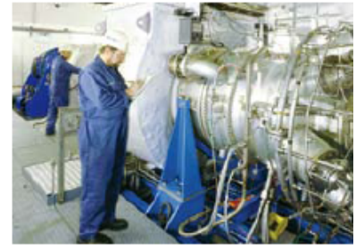
SGT-400 core engine test facility.
