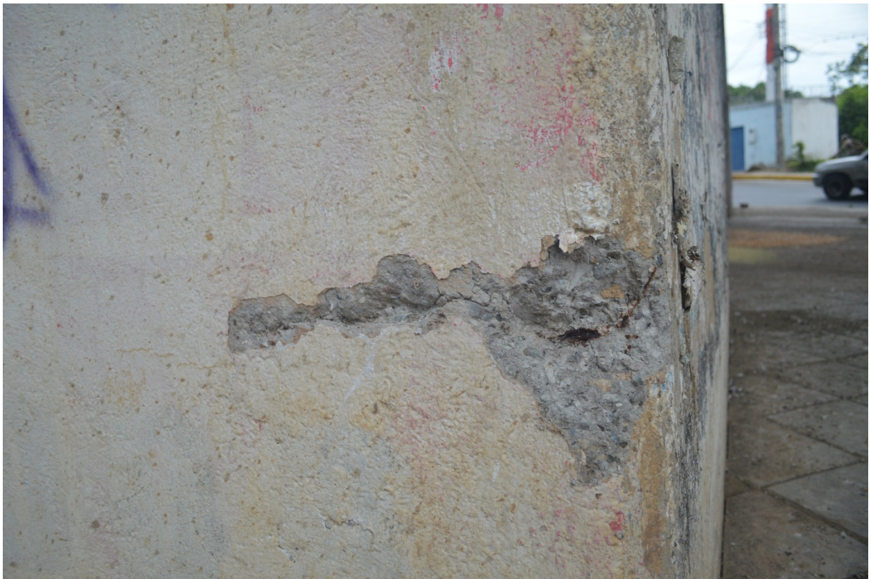
Figure 24. Environmental defects detected on the pier.
