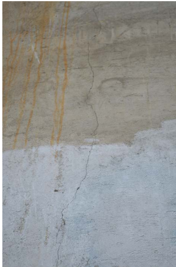
Figure 23. Small crack detected on the pier.
