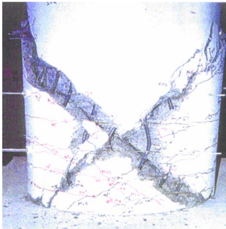
Figure 9. Diagonal crack (plastic hinge region-base). Adapted from Caltrans, (2006).
