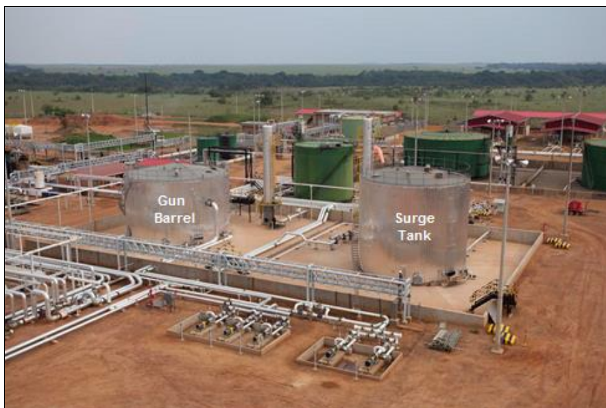
Figura 9. Surge Tank GB-2100 y Gun Barrel GB-2102 A/B.
