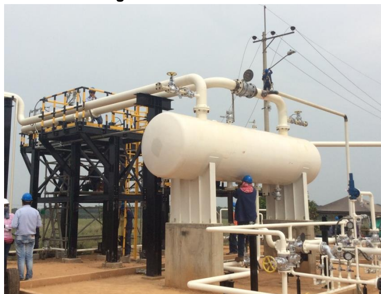
Figura 12. Knock Out Drum
