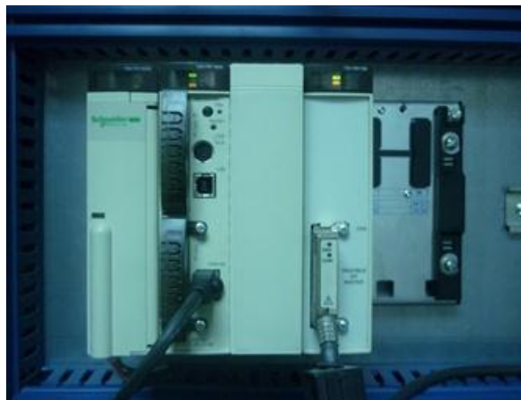
Figura 15. PLC Schneider TSX P57 4634.
