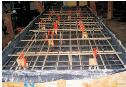
Fig. 1-The hybrid GFRP/CFRP (alternate bars) reinforced full-scale bridge deck slab is ready for placement of the FRC (0.5% V_f , 2” long fibrillated polypropylene fibers) matrix.
