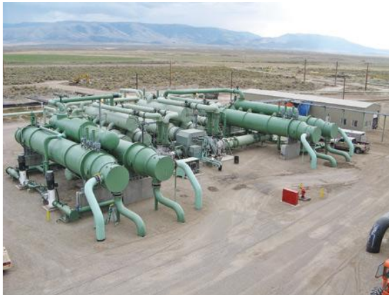
Figura 238 Raft River geothermal power plant
