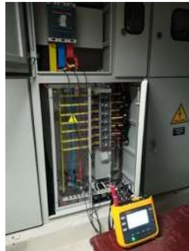
d) Fluke 1730 tablero general.
