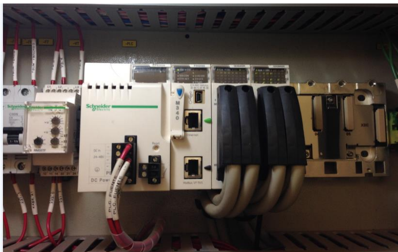
Figura 10. PLC (Programmable Logic Controller)
