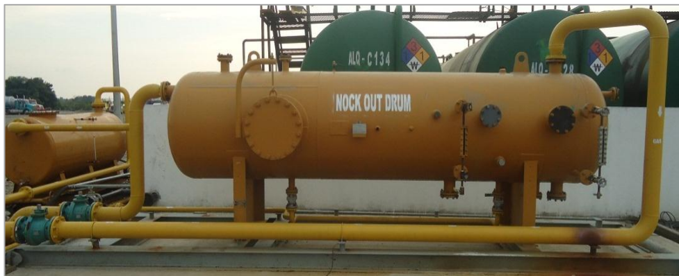
Figura 21. Knock Out Drum Horizontal
