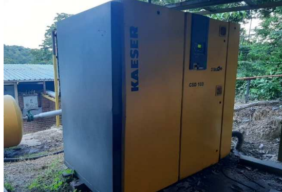
Figura 9. Compresor Kaeser CSD 100.
