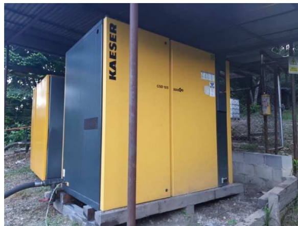
Figura 11. Compresor Kaeser CSD 125.
