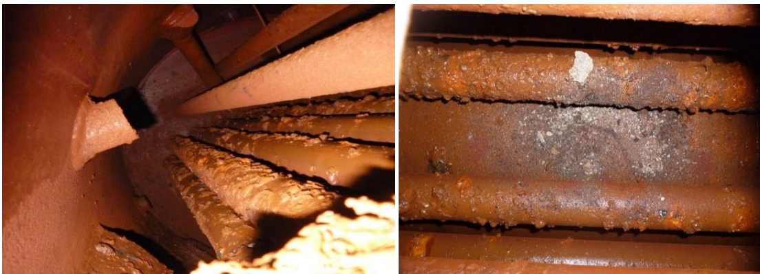
Figura 58. Detalle interior Hand Hole lateral.
