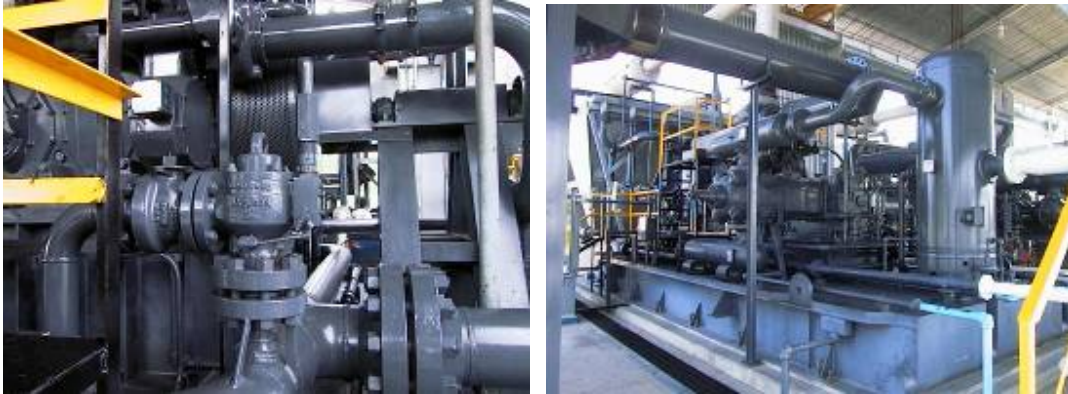
Figura 75. Safety Relief Valve (Unidad 1)
