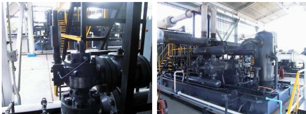
Figura 76. Safety Relief Valve (Unidad 2)
