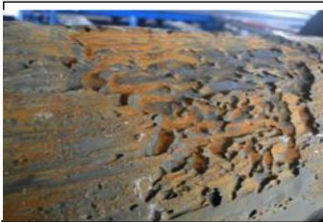
Housing's surface presented corrosion
