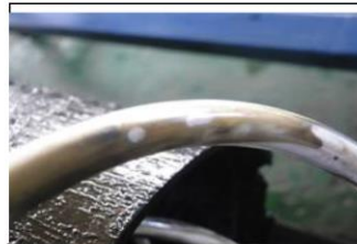
Top leads were found with water inside protection
