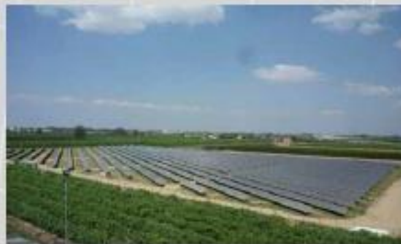
Free-field installation, Italy
