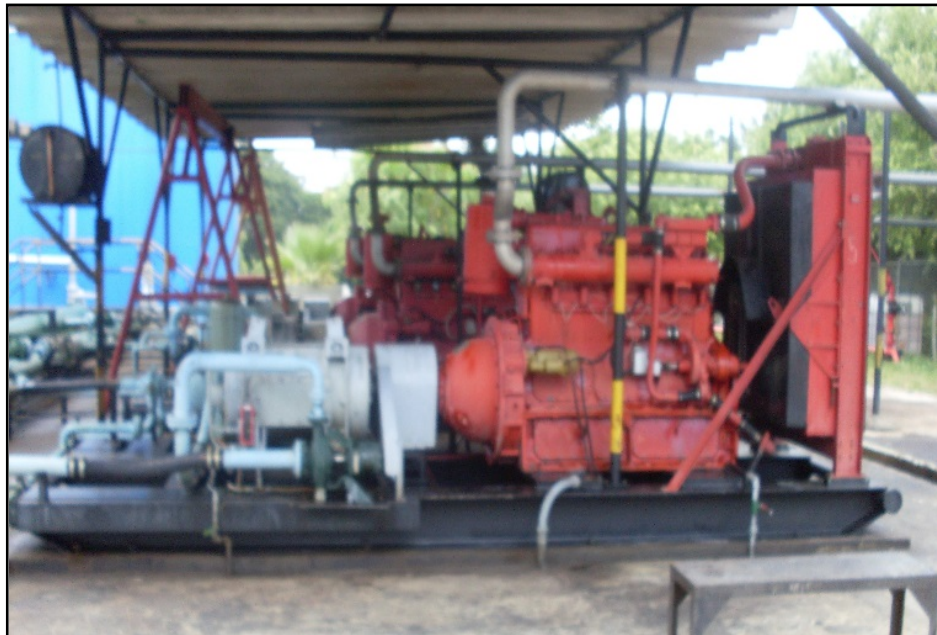
Figura 10. Bombas Kobe GS 1
