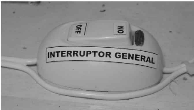
FIG. B3 INTERRUPTOR GENERAL
