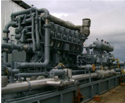
Figura 21 Moto Compresor Boosting Recetor
