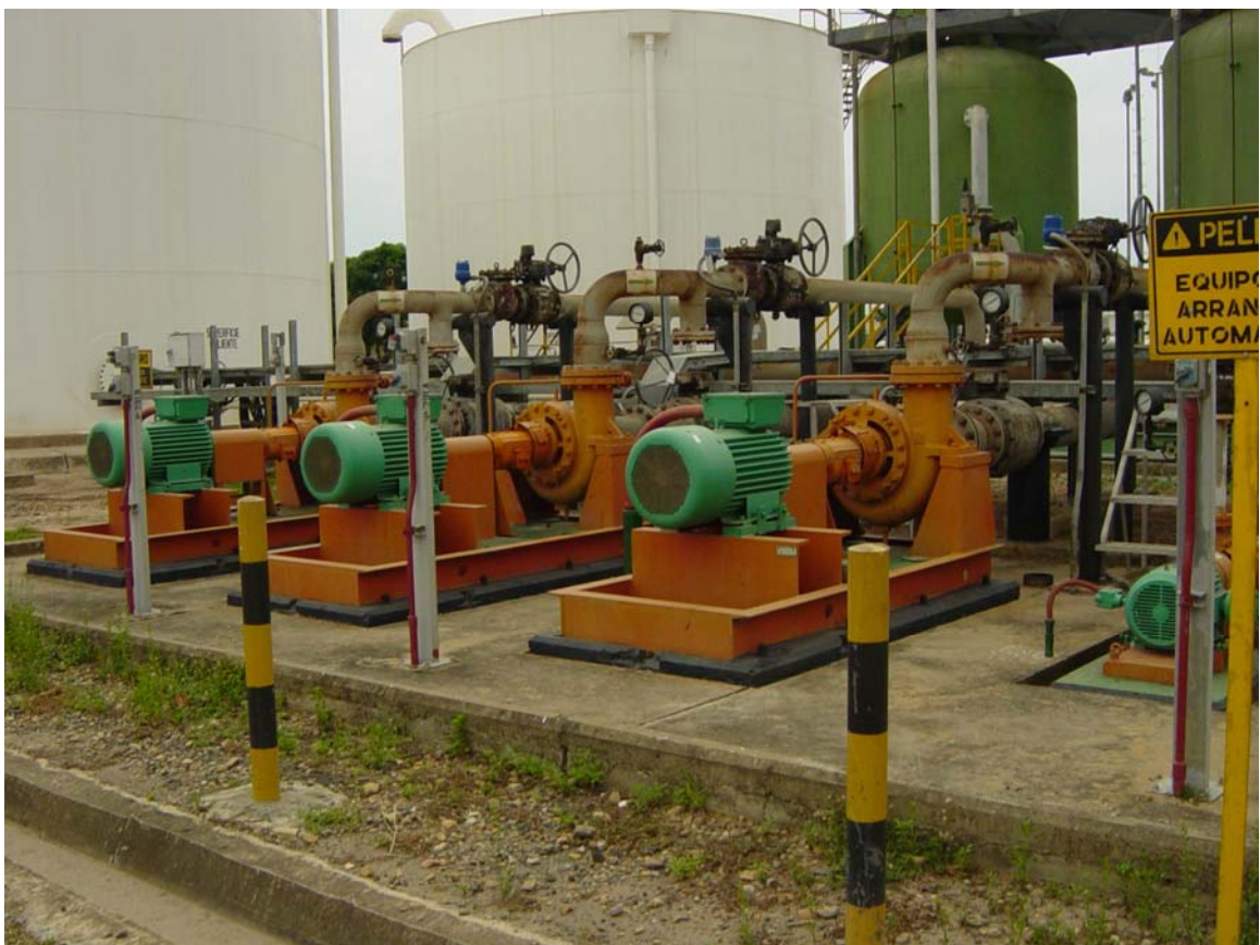
Figura 10. Bombas "Booster" P-791 A/B/C
