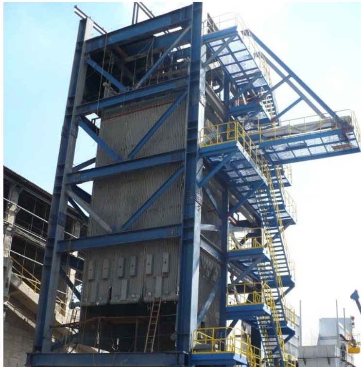
Figura 4. Caldera dedini AT 77
