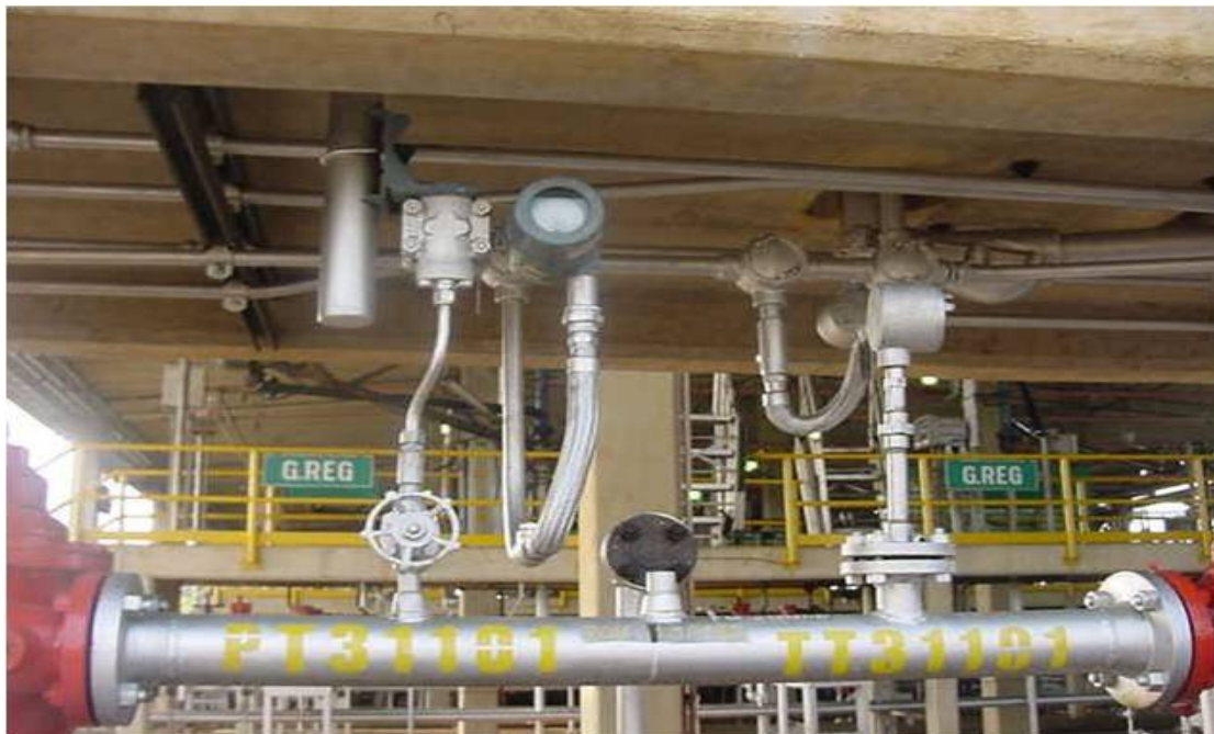
Foto 5. Pressure Transmitter Rosemount Inc. y Temperature transmitter Rosemount Inc.
