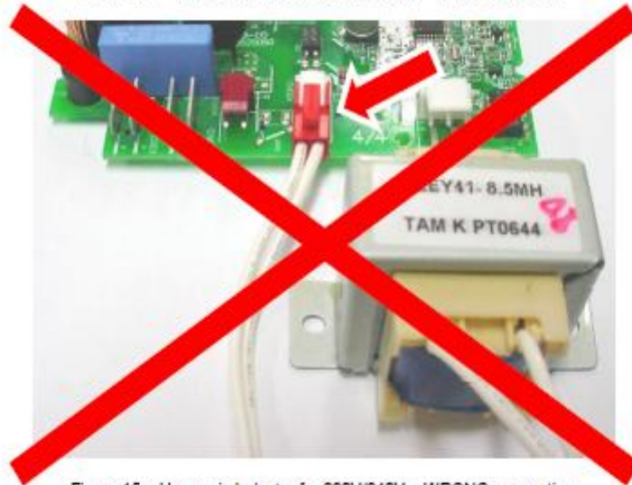
Figure 15 – Harmonic Inductor for 220V/240V – WRONG connection.
