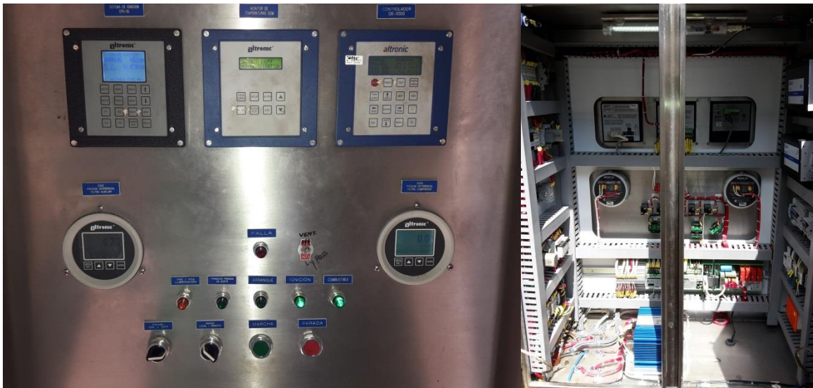
Figura 40. Panel de control motocompresor 04LP
