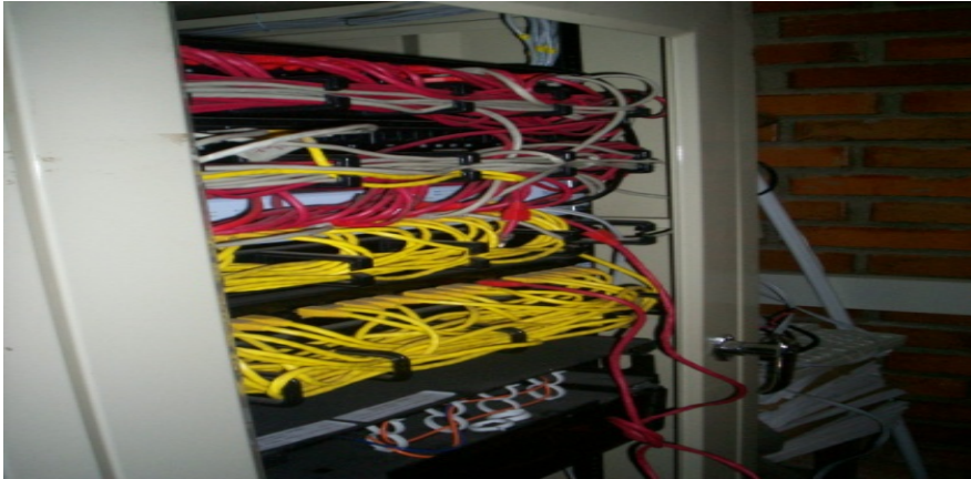
Figura 11. Rack Admon Control de Salas
