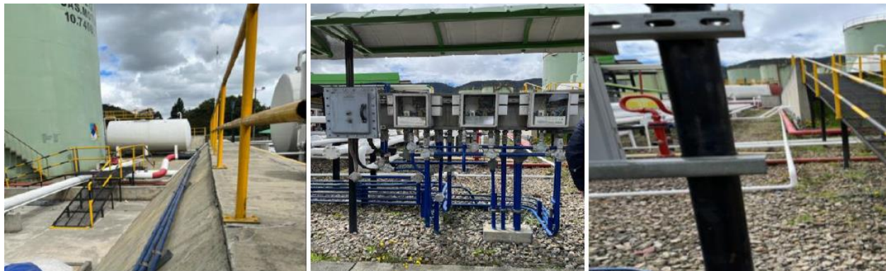
Figura 30 Hi Tracing Tanque 100 A B100
