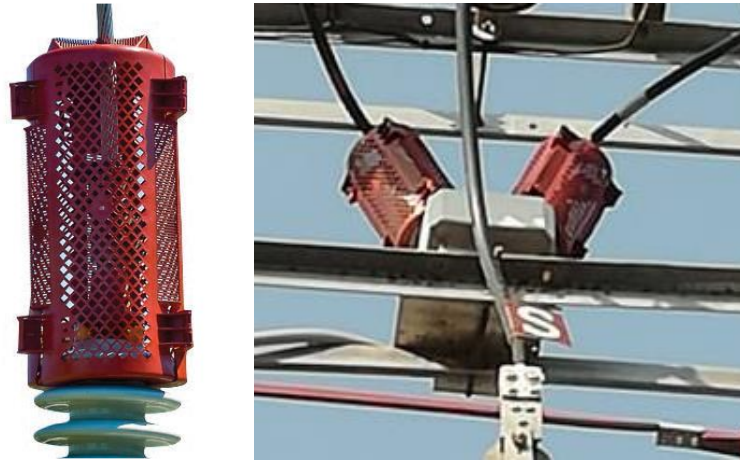
Figura 16. Bushing Connetion Inspection Cover; instalado en PT portico 22 en Cantagallo
