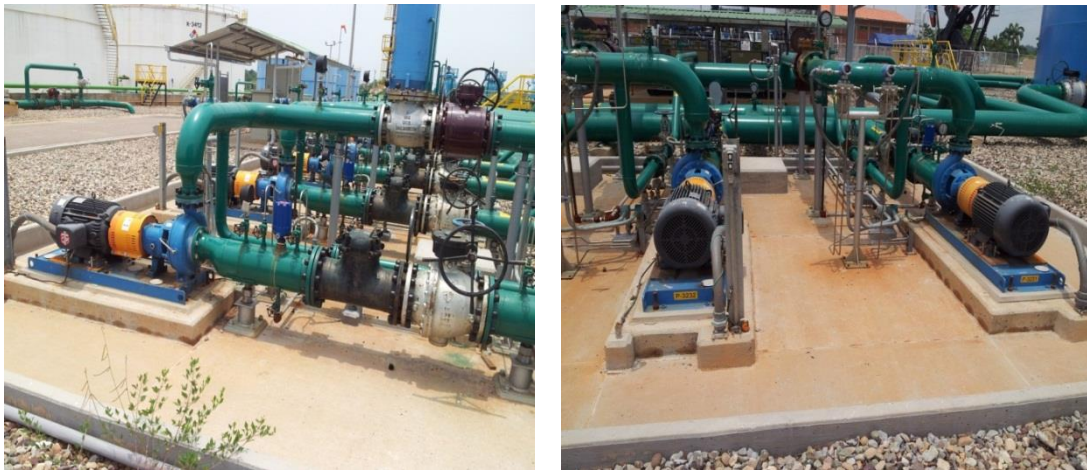
Figura 47. Bombas reforzadoras (booster) P-3231/32/33/34/35/36.
