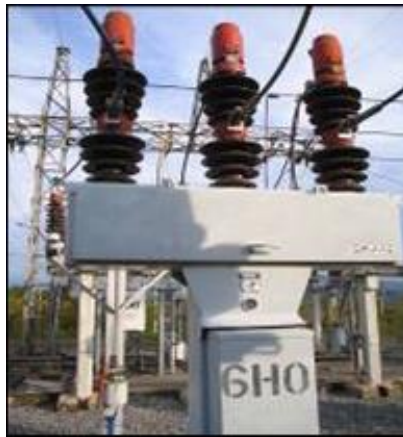
Figura 1. Interruptor CEM RGE 36-50-800 34,5 Kv
