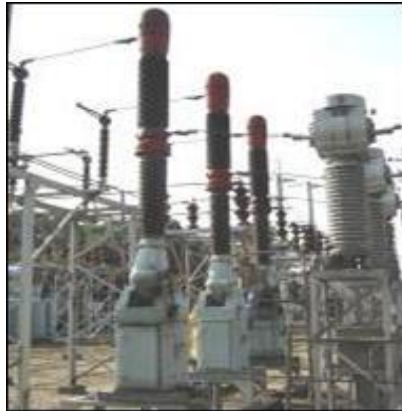
Figura 6. Interruptor DELLE ALSTHOM HPGE 11/15 E 115 kV
