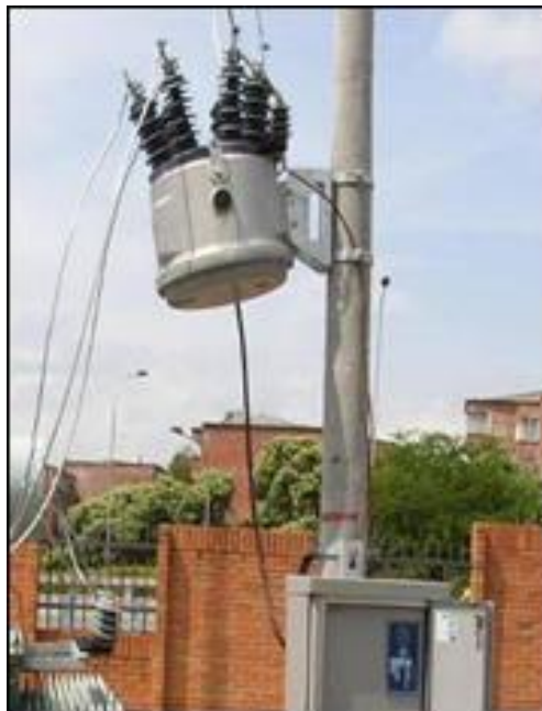
Figura 21. Recloser GVR 15 kV
