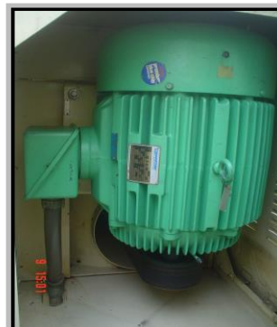
MOTOR ELECTRICO EXTRACTOR "A" CABINA TURBINA
